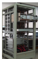
RF + Array Antenna
