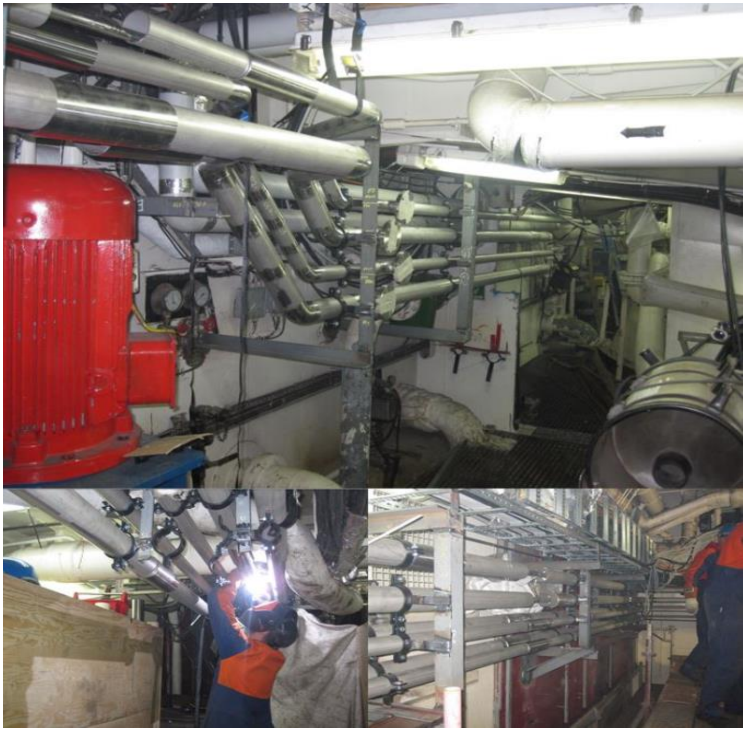
High pressure pipes
